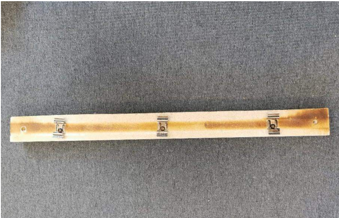
Photo No. 2 Damages on the wooden lath
